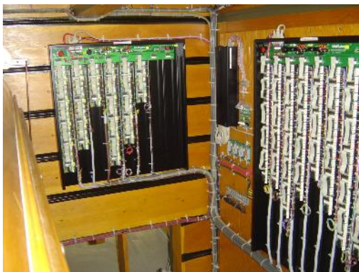
New Solid State control systems installed in the Austin AIRBOX.
